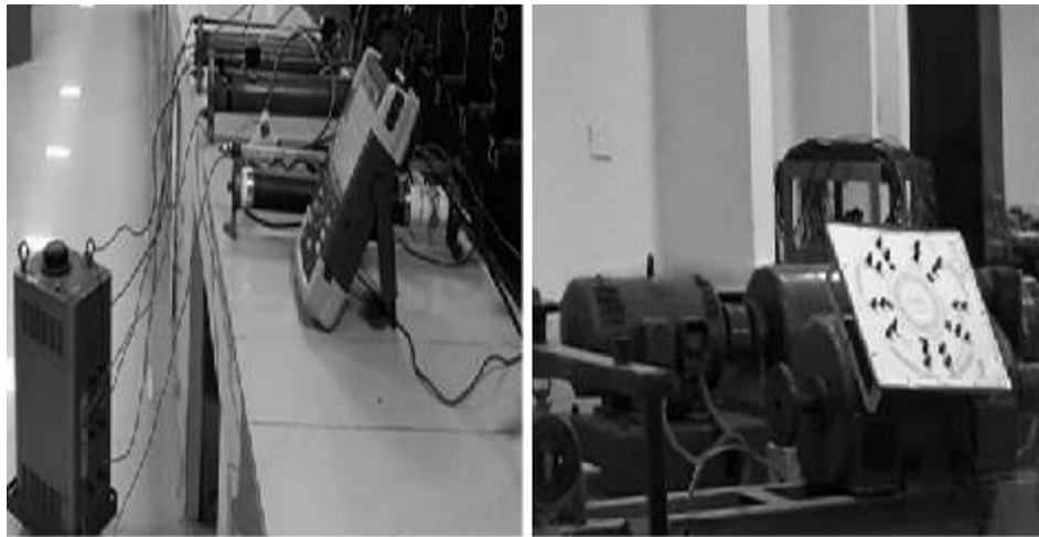
Figure 4: Experimental setup to identify stator related faults of induction motor
